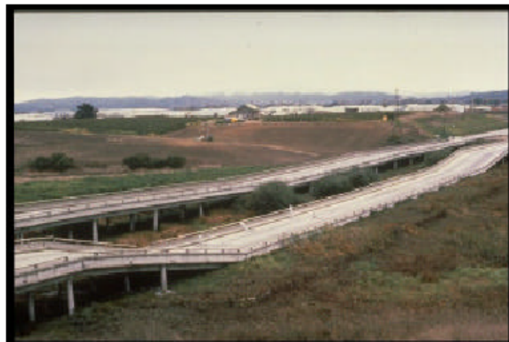
Figure 2.5 Highway 1 Crossing Struve Slough near Watsonville Collapsed during the 1989 Loma Prieta Earthquake, with Pile Punching through Deck (after Seed et al.,1990)
