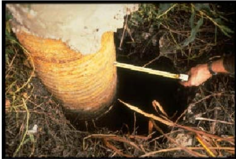
Figure 2.6 Formation of gap adjacent to one of the piles supporting collapsed Struve Slough Crossing during the 1989 Loma Prieta Earthquake (Seed et al.,1990)
