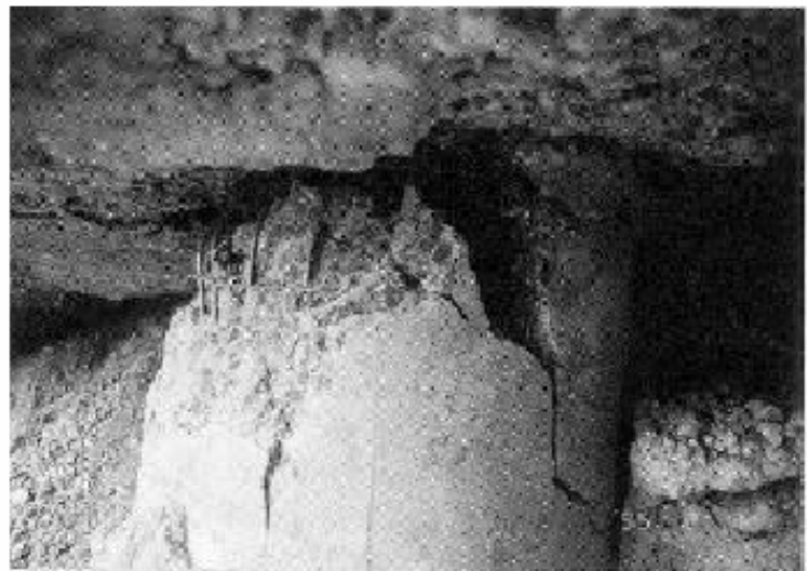
Figure 2.10 Lateral spreading damage to pile during the 1995 Kobe Earthquake (after Tokimatsu et al., 1996)
