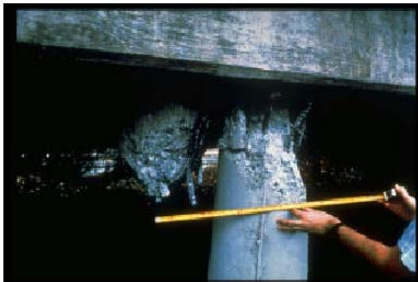
Figure 2.7 Flexural shear failure of pile to bent connection of the Struve Slough Crossing during the 1989 Loma Prieta Earthquake (Seed et al.,1990)
