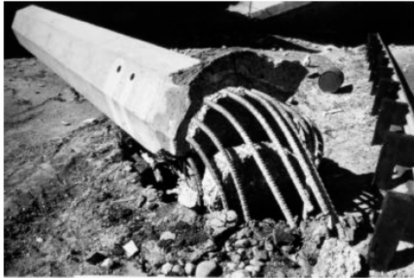
Figure 2.3 Failure at connection detail between drilled shaft and bridge column at the Golden State Freeway/Foothill Freeway Interchange during San Fernando Earthquake (after Penzien, 1971)
