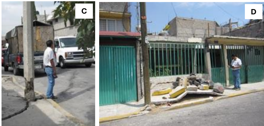
Gambar II. 9 Dampak Land Subsidence di Kota Meksiko ( Hidrologi Group. FIU Geodesi Lab in in Tzampoglou et al., 2023)
