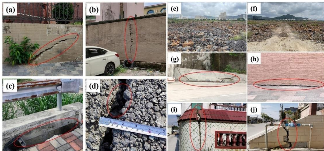
Gambar II. 1 Contoh Dampak Kerusakan Land Subsidence (I) (Liu et al., 2023)
