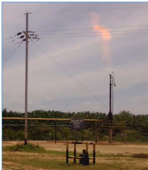
Figure 1.4. Flare Stack in Beta Station
