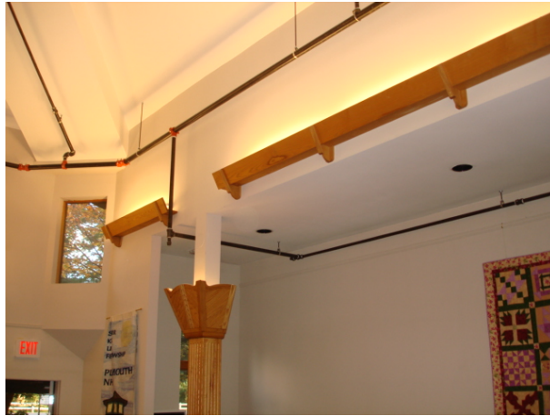
Gambar II.9 Sprinkler di AVA Gallery, New Hampshire Sumber: www.ironworksfire.com , diunduh 11 November 2014
